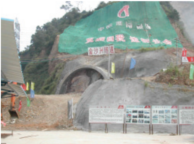
Bild 6. Nordportal Jinsha Zhou Tunnel, Baubeginn 2006 Fig. 6. North entrance Jinsha Zhou Tunnel, beginning of construction 2006
